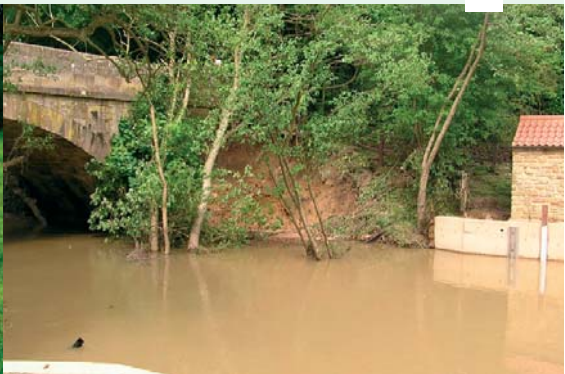
Figure 4. The bridge down stream from Hawnbly, closed due to undercutting of the stone parapet. Note the flood gauge in the river, although the floodwaters topped the gutters of the adjacent flood gauge building.
