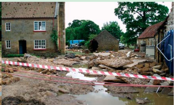
Figure 2. Damage to farm buildings and cars washed downstream at Boltby. Note the 'tide mark' of floodwaters just below the ground floor windows. Gurtof Beck is located a few metres to the right of the outbuildings. Photo: Pete Hobbs/Helen Reeves. (BGS)
