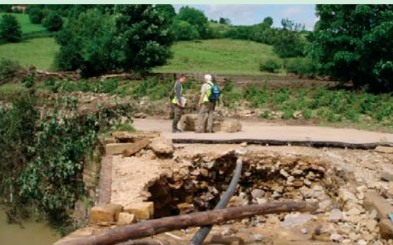
Figure 1. Flood damage to the bridge at Hawnby. Note the brown 'tide mark' (arrow A) of debris in the middle distance indicating the level of the Rye floodwaters; this coincides with the mapped alluvium boundary on the geological map. The dashed arrow indicates the direction of flow and a flatted field of small conifers. Photo: Pete Hobbs/Helen Reeves. (BGS)
